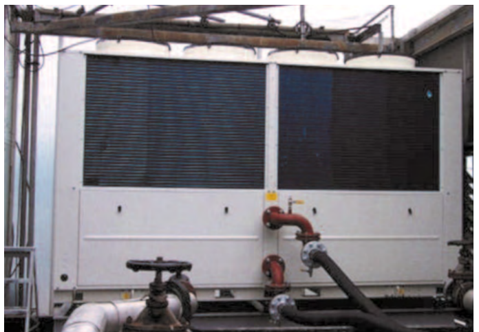
The newly installed YLCA chiller unit
